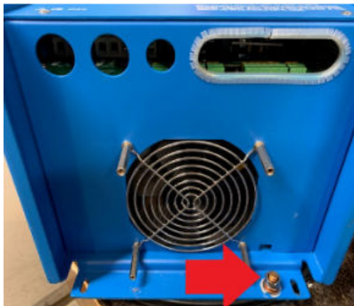
Figure 26 - 3kVA Ground Connection Point
