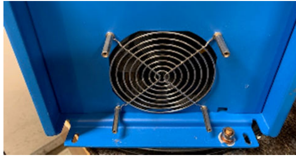
Figure 5 - 3kVA Blue Fan Cover Plate Removed
