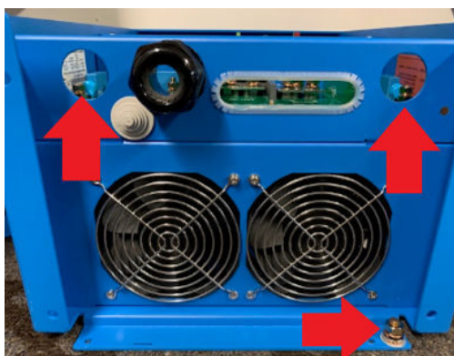
Figure 27 - 5kVA Ground Connection Points
